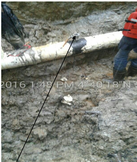
2" Valve installed by vandals
